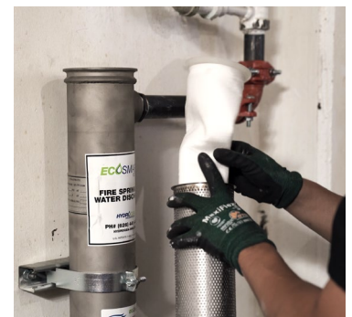
The smaller wall mount EcoSmart Filter unit is installed near the inspector's test location
